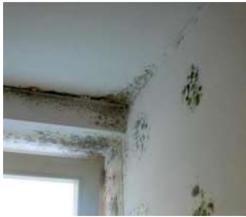
Fig. 1 Concrete wall attacked by mould
