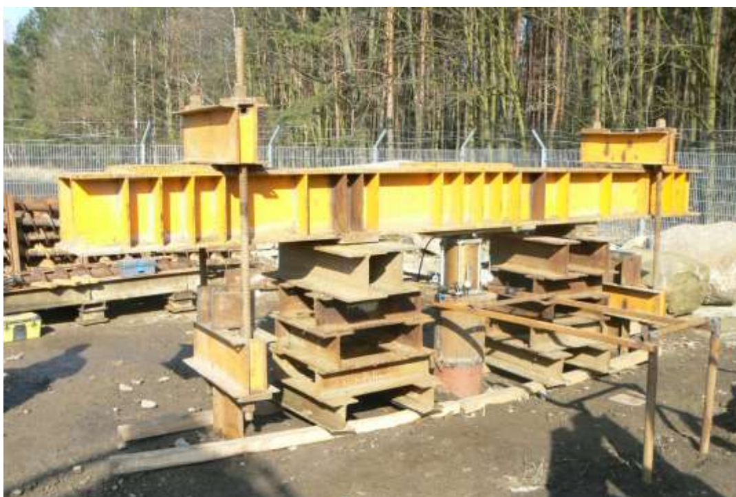
Fig 1. Static load test of tubular cross steel pile with reaction system anchored to two jet grouting piles.
