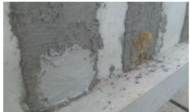
Fig. 3. On the right side PBO fan before applying the mortar, on the left after the mortar application
