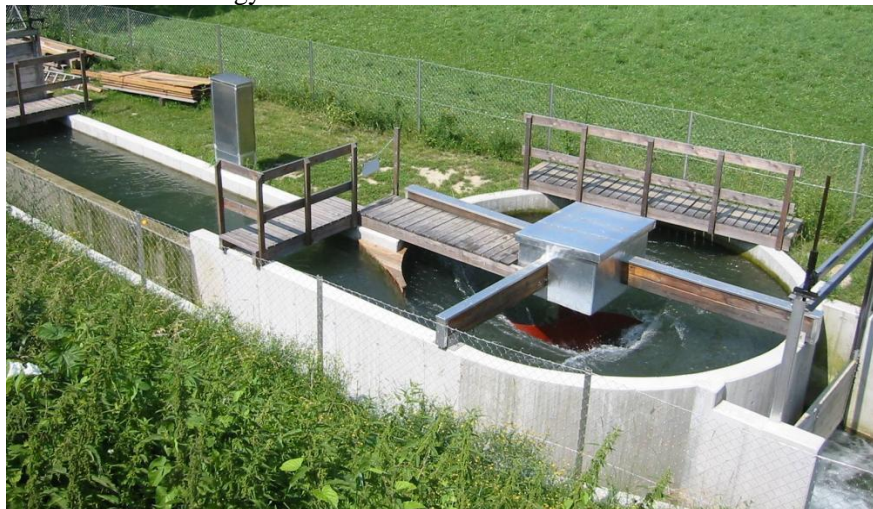
Fig.2. Micro-hydroelectric power station
